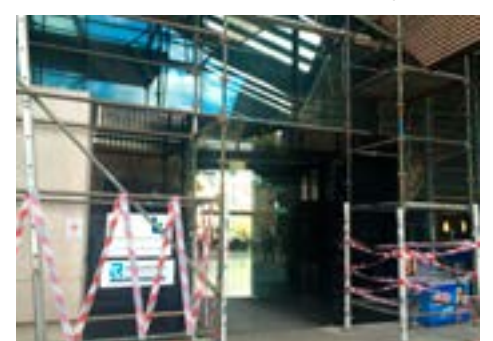
The ERC. Also under construction. Perhaps they're removing the old student centre.
